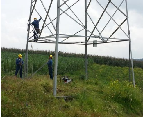
Figure 3. Tower without redundant members (stolen).
