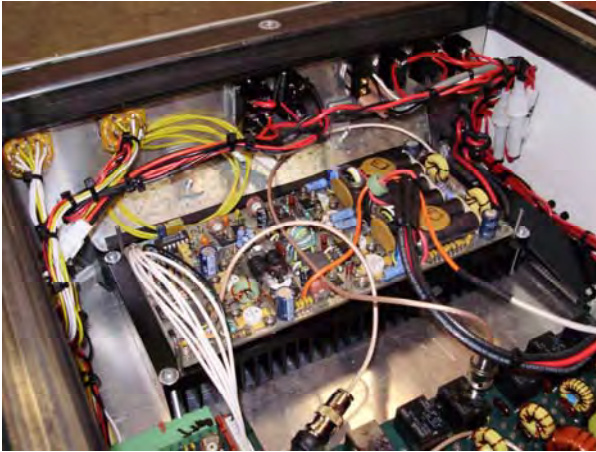
Figure 2. Amplifier and heat sink inside cart, near duct.
