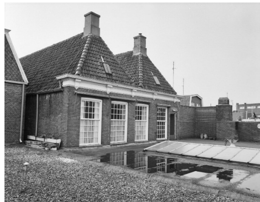
Figure 1. Back side of the first floor of the Hofkeshuis (the annex on the ground floor is a modern addition). The first three windows from the left are those of the rear salon (photo: Cultural Heritage Agency of the Netherlands (RCE), 1974).
