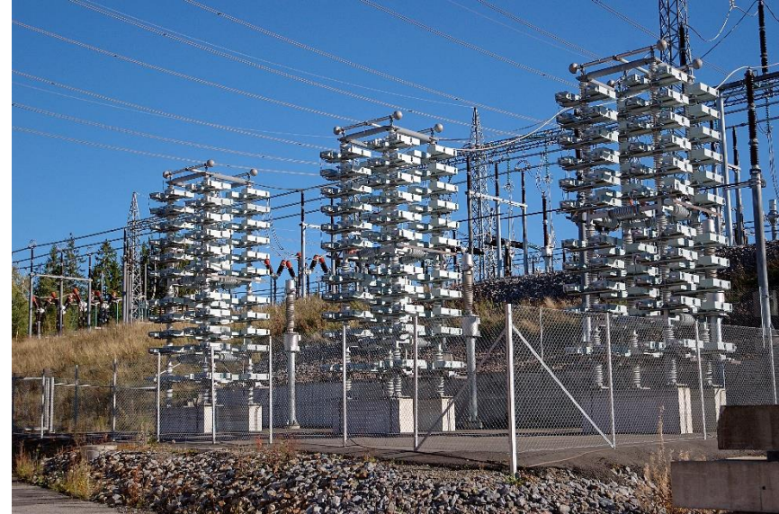
ABB shut capacitor bank
