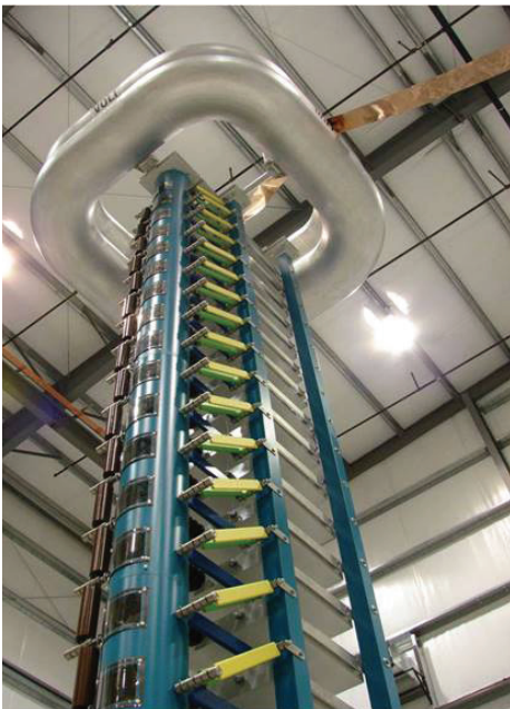
FIGURE 1. High-voltage generator (2.4 MV Marx generator) operated by NTS.
